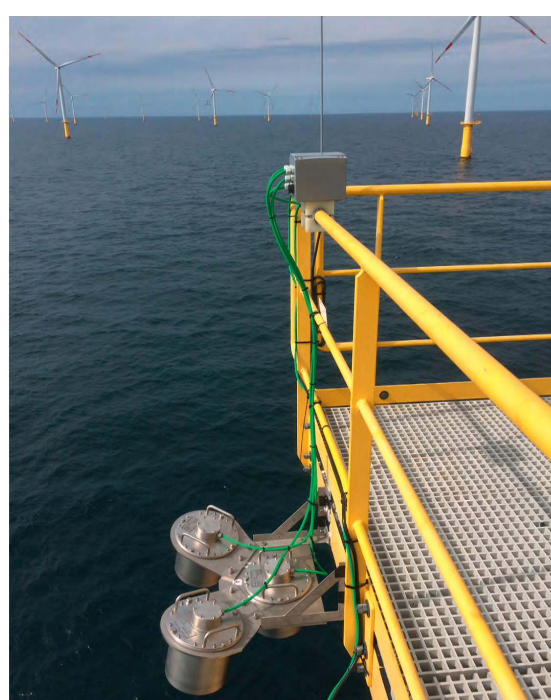
Fig. 2: Directional sea state radar at wind farm Butendiek.
